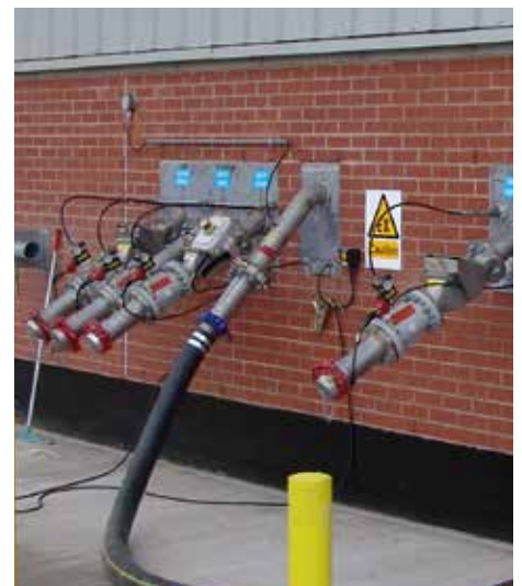
Pneumag installed at bulk material intake, ATEX rated.
