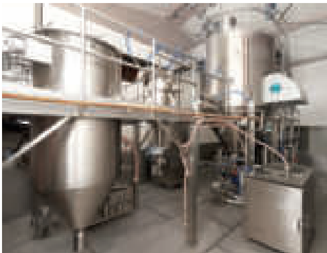
Pilot plant with homogenizer and safety equipment
